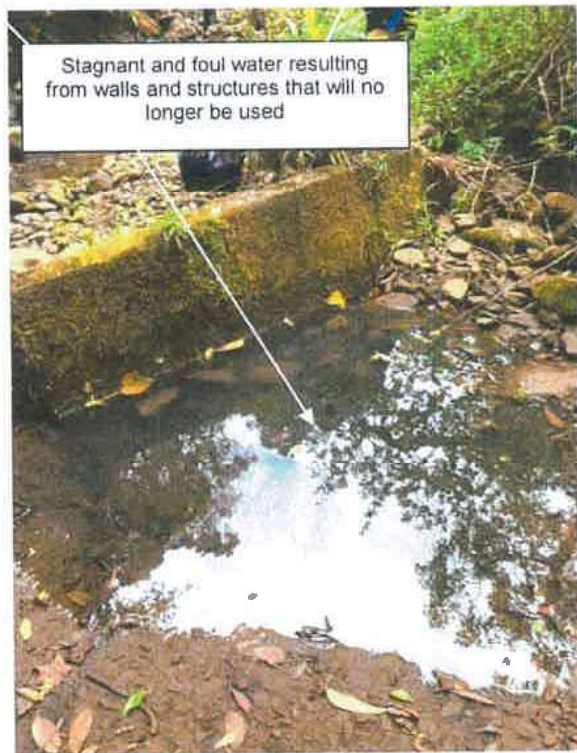
Figure 4. Stagnant water standing in depressions created by the walls and the gate structure.
