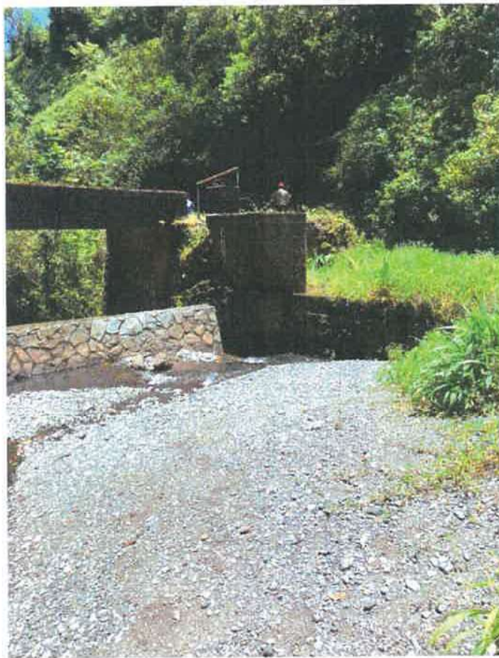
Figure 11. Dam, gate, and control structure at K-21.
